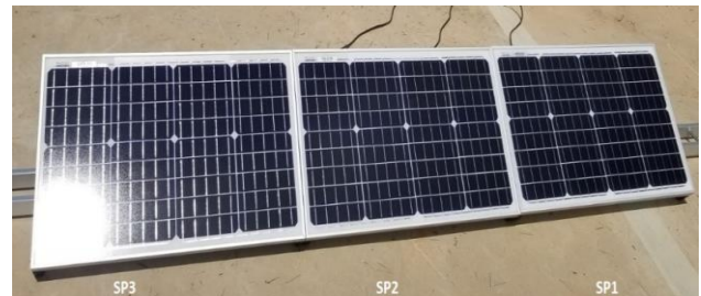
Fig. 1. View of solar panels in string
