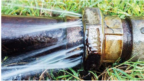
Fig. 2. Leakage in pipes
