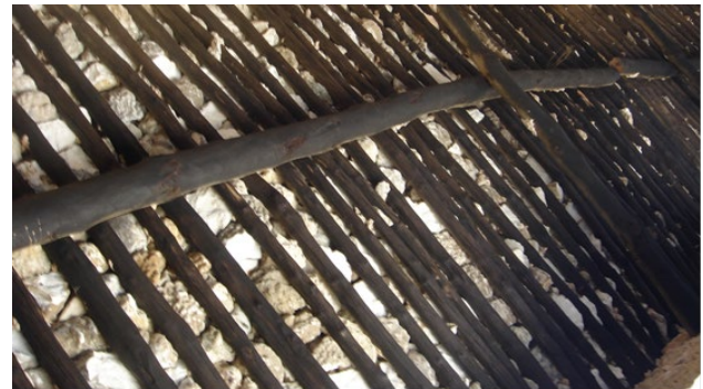
Fig. 5. The mangrove poles ceiling in the contemporary Swahili house in Kilwa Kisiwani
